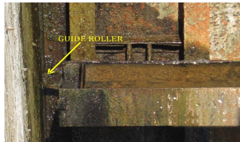
HEAVY RUSTING DUE TO LEAKAGE OF
