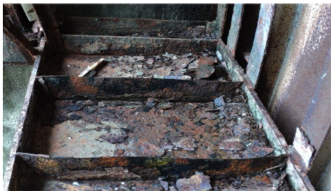
A GATE COMPONENT HEAVILY RUSTED WATER
