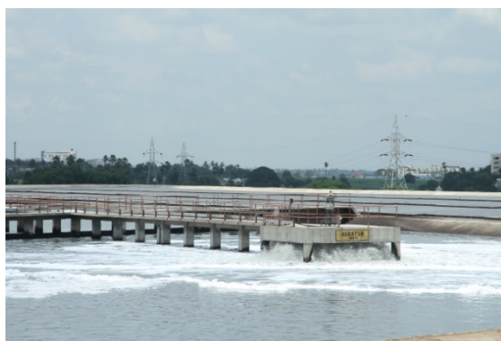
Extended Aeration System in Amberpet STP
