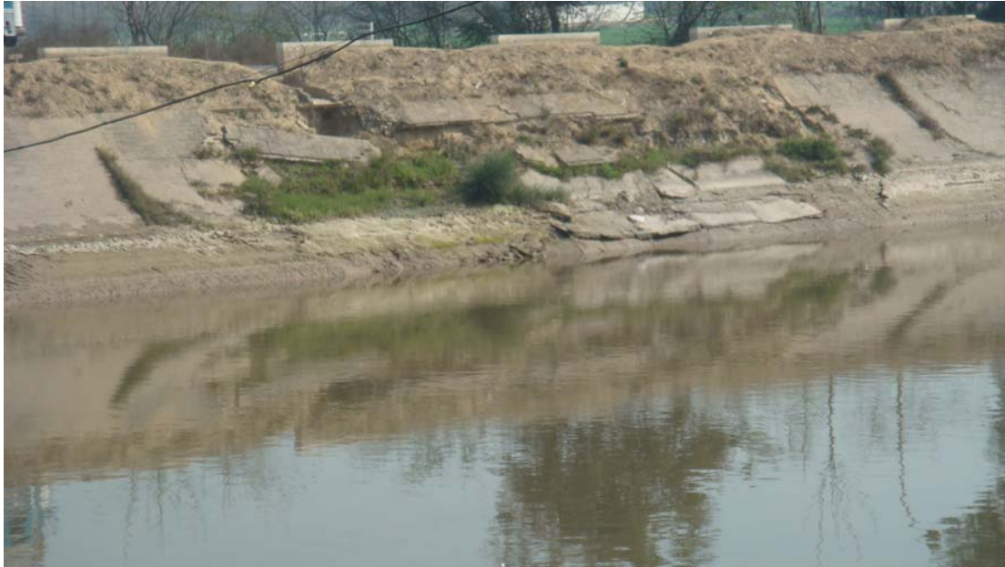
Photograph 1. Damaged lining of Rajasthan Feeder
