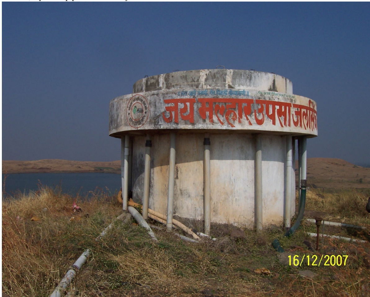
Photograph-1 shows Main Distribution Chamber and vertical pipe carries water to Small Distribution Chamber
