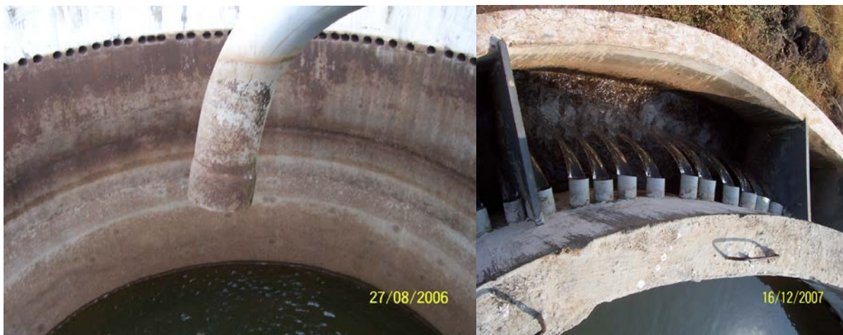
Photo no. 4 shows Equal Diameter Pipes fixed at equal distributing equal quantity of water
