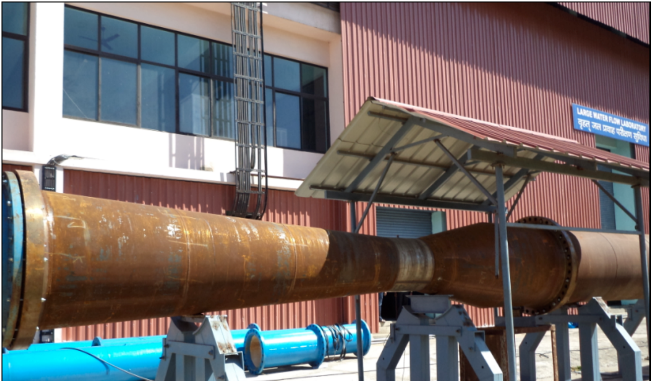
Photo 2: 1000mm Venturi Flow Meter Under Calibration
