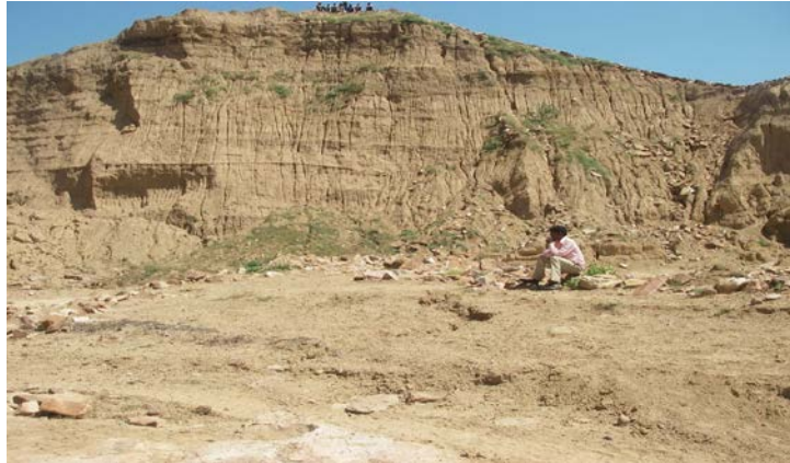
Fig 3: Breached section showing no visible signs for confirming the presence of chimney filter
