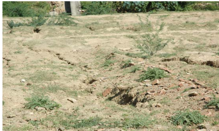
Fig 4: Downstream slope showing deep rain cuts and excessive weed growth
