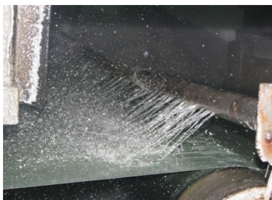
Fig 3: Inefficient Hole Showers consuming more water
