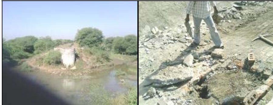
Photos – 3 and 4 Leakage and Identification of Piping through Banks
