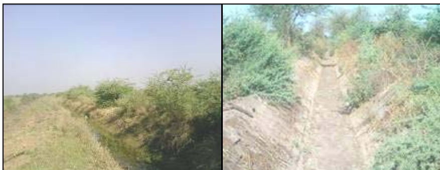
Photos - 1 and 2 Bad Condition of Tanchha Distributary
